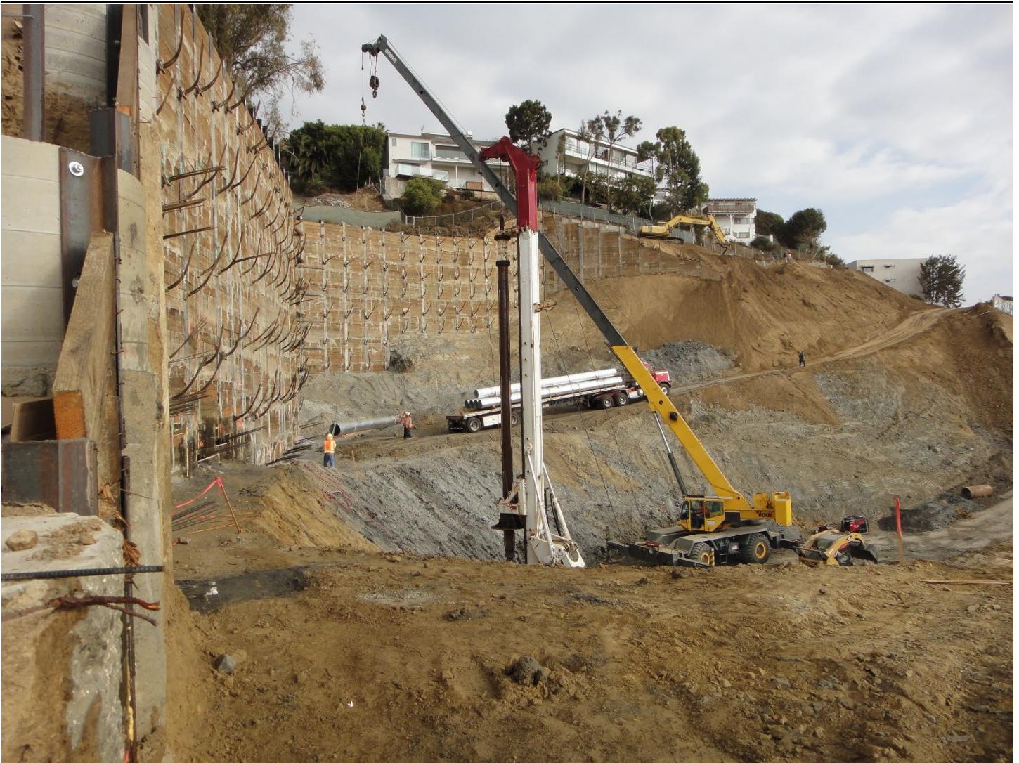
Photo 11: A major landslide repair in progress using grading, soldier piles and retaining walls.
