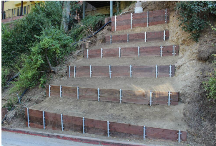
Photo 9: A surficial failure repaired using the pipe-and-board method.
